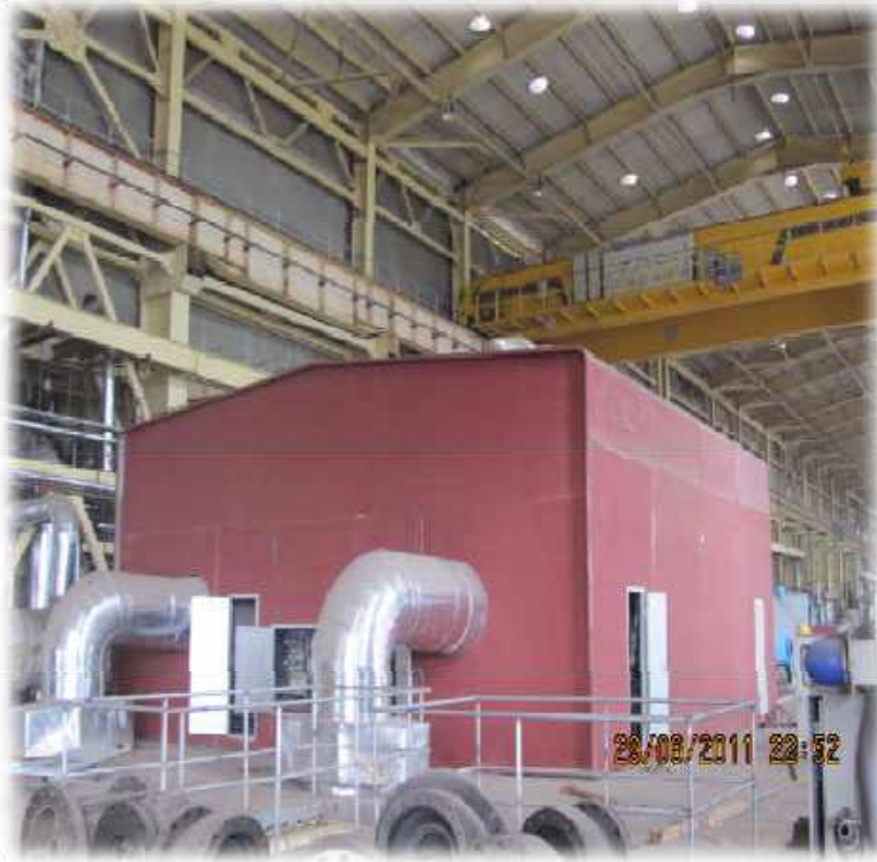
Turbine Generator III
