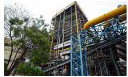
View of Boiler, Vijayanagar
